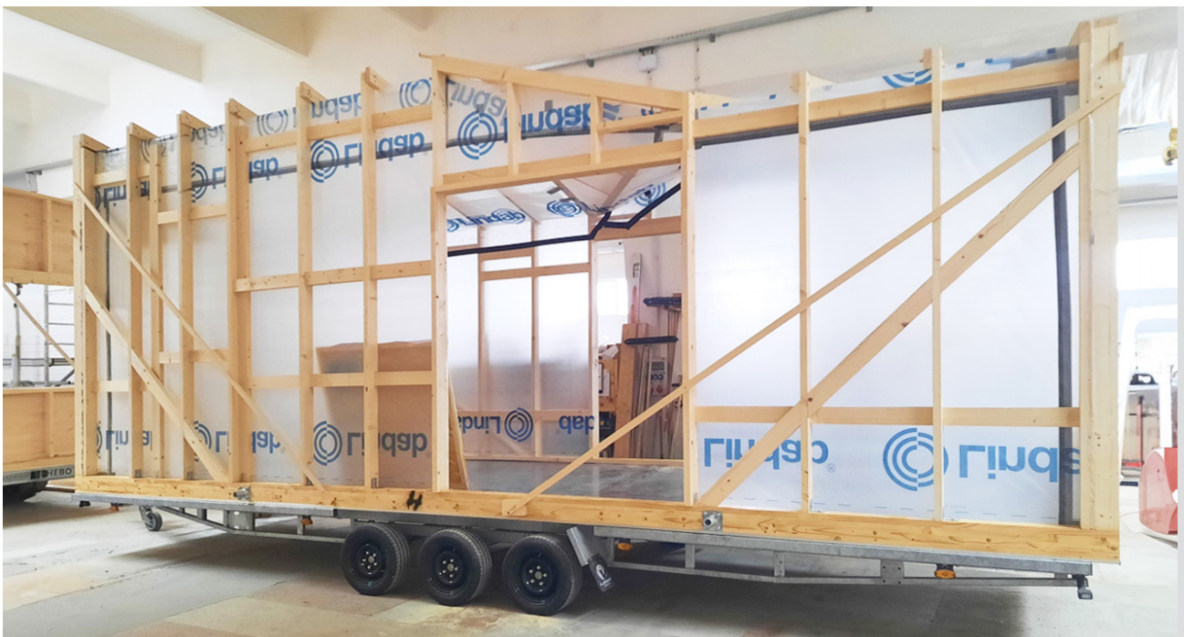
Fig. 2: The house is prefabricated off-site before being transported to its destination. Source: Kasawoo, 2024.
